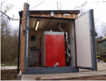
Biomass heating boiler installation at Torlundy.
